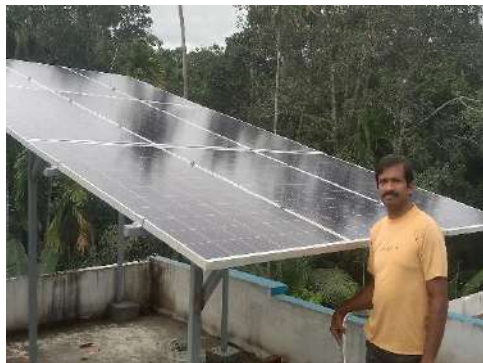
Arbin Joseph 3 kWp
