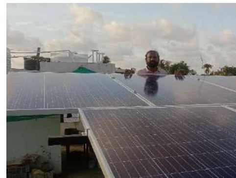
Alexander Thomas 3 kWp
