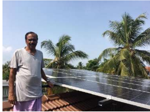
Moosa Uppunnikuzhi 3 kWp
