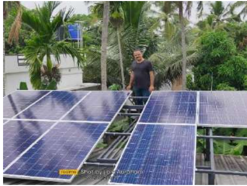
Madhusoodhan M.P 3 kWp
