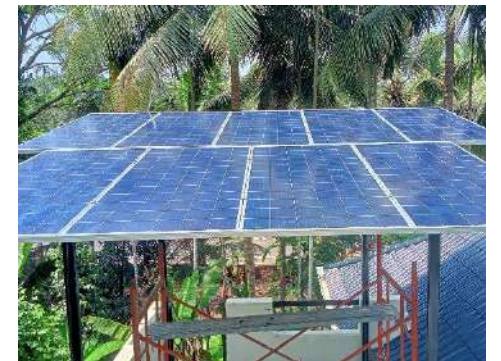
Mathewkutty M A 3 kWp
