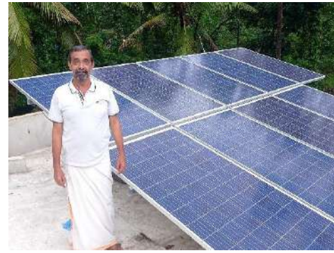
Sasi V.S 3 kWp
