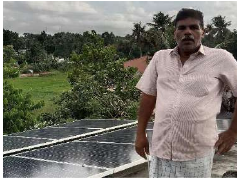
Basheer K.S 3 kWp
